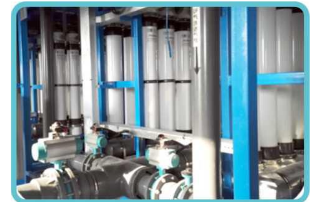
Desalination water treatment project
