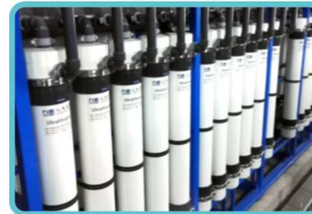
Papermaking wastewater treatment project
